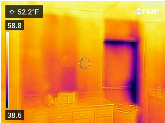
Image 2-3: (This is an image of a basement door connecting to the exterior. This door is leaking cold air around the frame- the purple color.)
