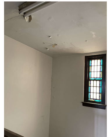
9 - Paint chipping on ceiling
