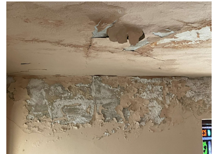
26 - Water damage and paint chipping on wall and ceiling
