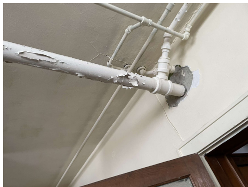
20 - Paint chipping on pipe
