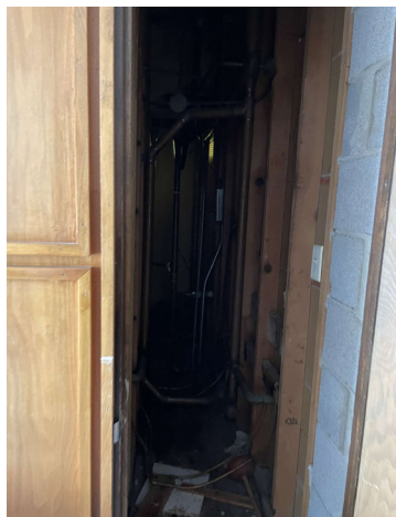
37 - Mechanical closet, pipes
