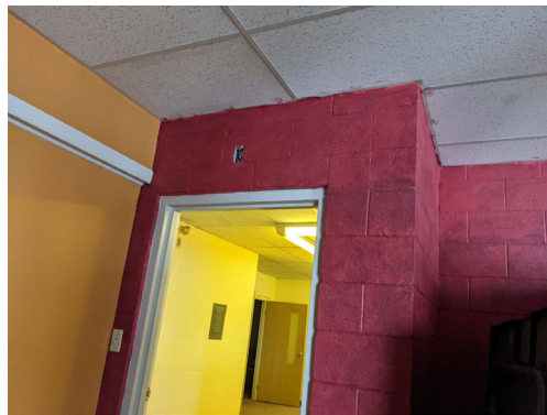
18 - Poorly painted wall (spots on ceiling)
