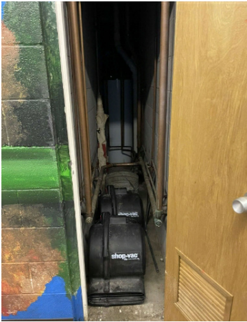
33 - Mechanical closet, generators
