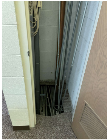
34 - Mechanical closet, pipes
