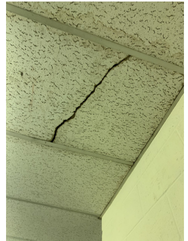
3 - Cracked ceiling tile
