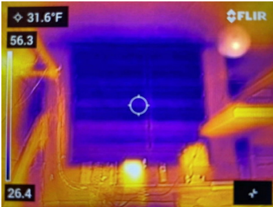
TC-1 - This is a garage type door in the basement next to the boiler room, showing a large amount of heat being lost through poor sealing and no insulation on the door. Although this room does not necessarily need heated it will lose common room heat if the door to the boiler room is left open
