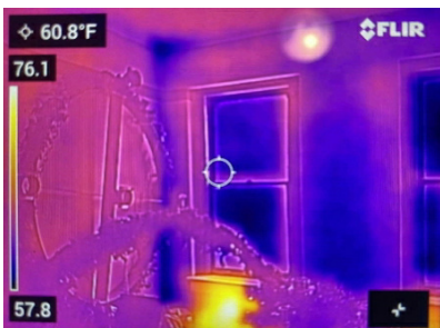
TC-17 - Another upstairs storage room shows extensive insulation damage and possible water damage down the corner of the wall.
