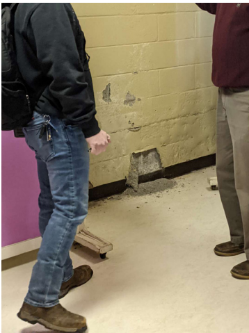
14 - Rotting concrete wall
