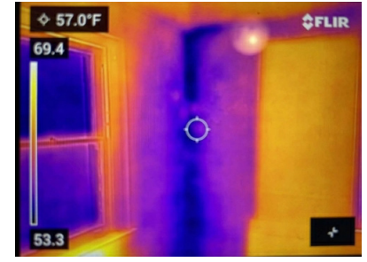
TC-13 - With a closer view of the corner, it becomes clearer that there is water damage in the wall. This should be addressed, or it will lead to more deterioration and a more costly fix in the future.
