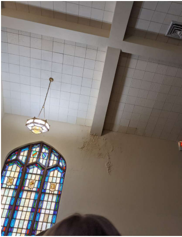
21 - Water damage in sanctuary
