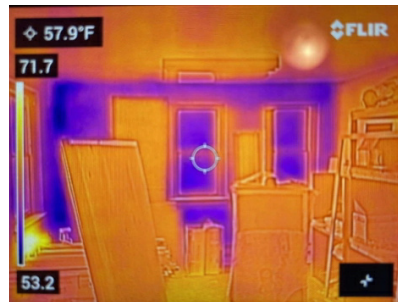
TC-15 - More missing insulation in an upstairs storage room. Renovation becomes more of a necessary decision throughout the process locating multiple rooms losing heat and driving the heating and cooling bills up.
