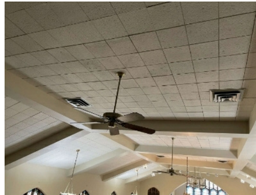
5 - Ceiling - water damage
