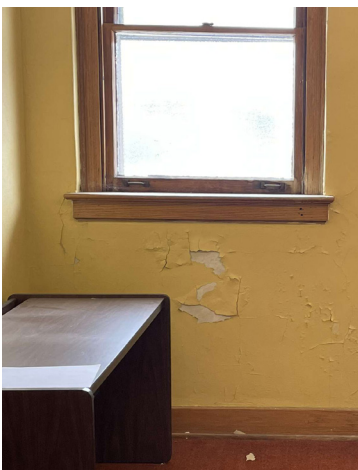
17 - Paint chipping on wall
