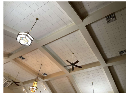
29 - Lighting in sanctuary
