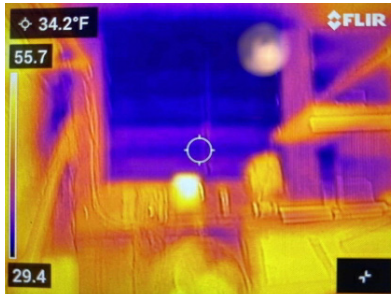
TC-2 - Garage door near boiler room - poorly sealed, losing a lot of heat
