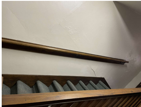
15 - Stairwell with cracked wall
