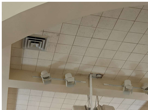
10 - Water damage around ventilation
