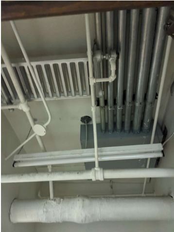
11 - Pipes on ceiling
