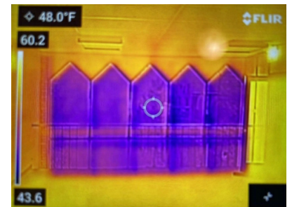
TC-6 - The blue color of the windows isn't necessarily an issue because heat will inevitably be lost through this glass. Although, this thermal reading does make it apparent just how much heat is lost through these windows. It may not be visually appealing but replacing these windows with a wall the church would save money on heating and cooling.
