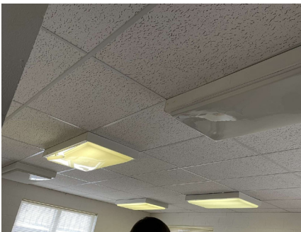
27 - Broken luminaires, burnt-out lamps
