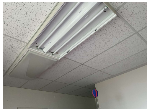
31 - Luminaire with missing cover
