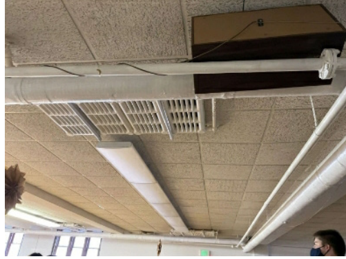
12 - Cords wrapped around pipes
