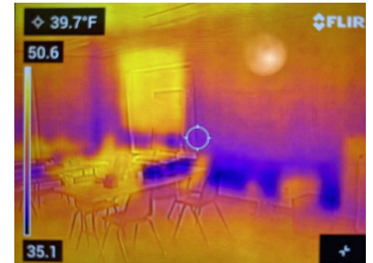
TC-3 - Heat is lost through the baseline of the wall this could be due to many things including poor insulation. This is not a single occurrence many rooms have one or multiple walls with this issue costing the church money in heating and cooling during the summer.
