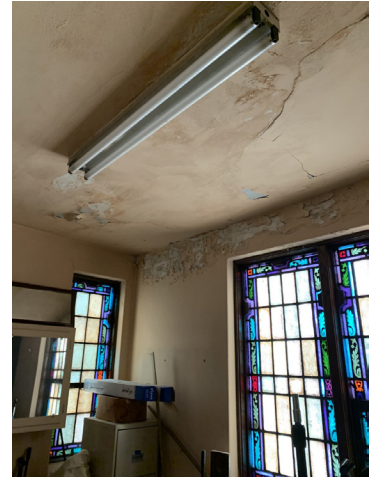
13 - Water damage on ceiling and wall
