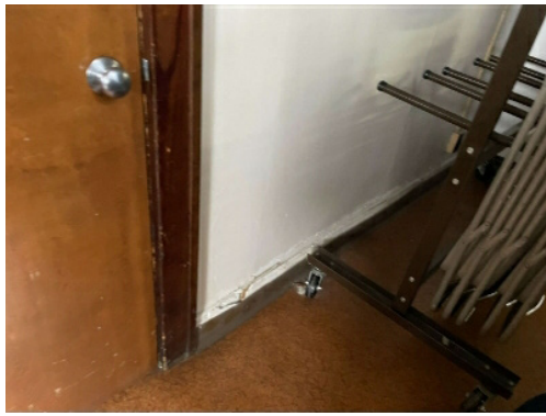
25 - Water damage on trim
