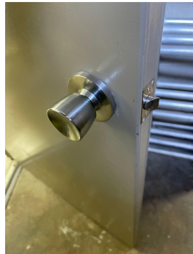
Door knob to room with electrical panels - does not have a lock so anyone can open it at anytime
